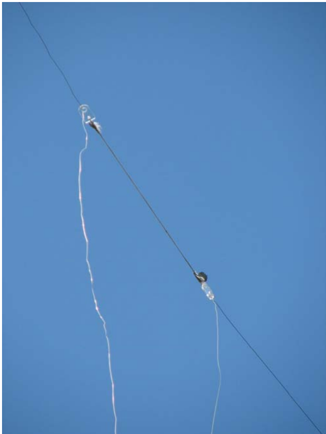
End of the vertical part, 80m inverted L left, 160m inverted L to the right, both with plexiglas insulators connected with Dyneema rope.
